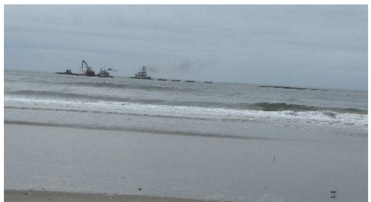
Figure 2. Boats and a pipe from a dredging operation off Atlantic City. Photograph by Don Nigroni
